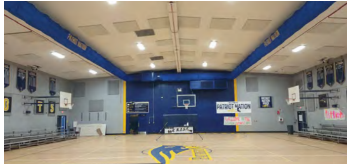
Thomas Jefferson Middle School HVAC, Madera Unified School District
